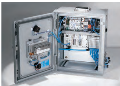
Custom Control Cabinets Comprehensive engineering support and on-site services
